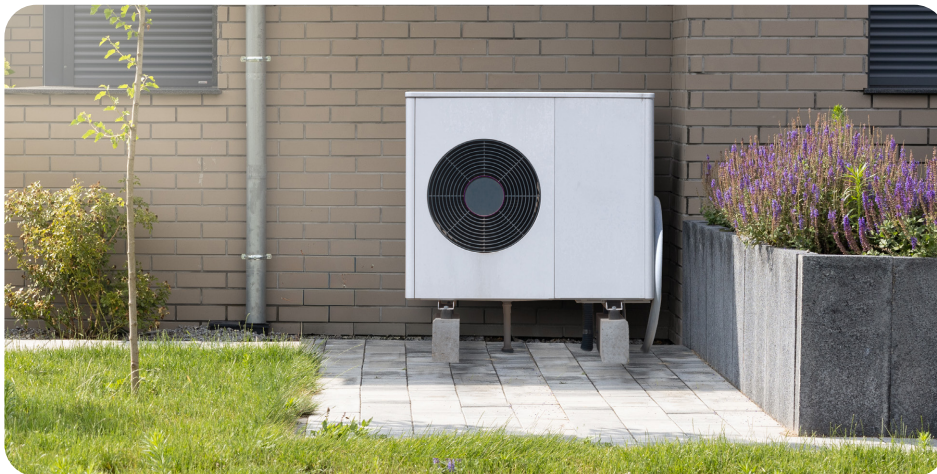
Modern heat pump system (Credit: Maxshot)
