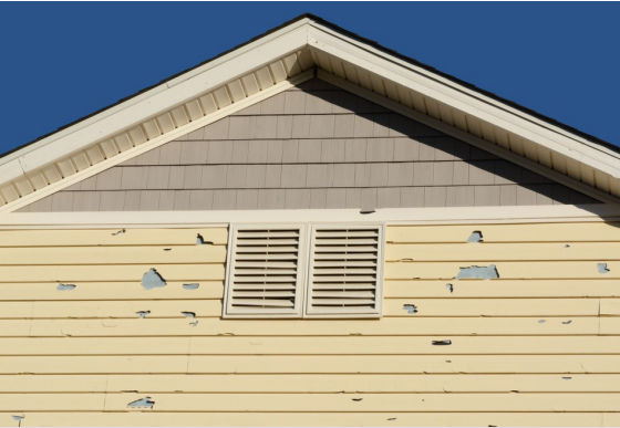
Siding damage from hailstorm.
