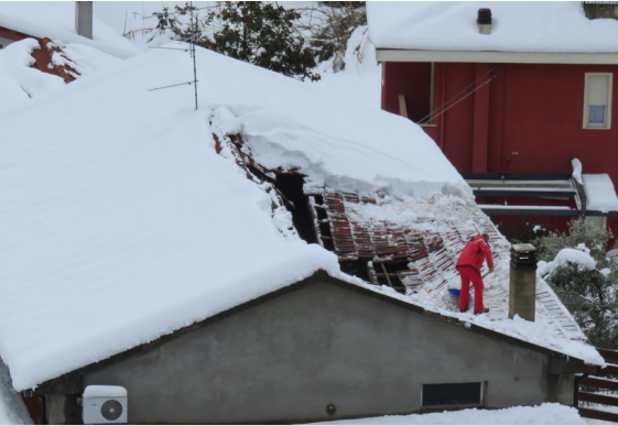
Roof collapse due to heavy snowfall.
