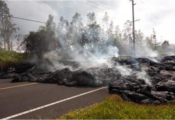
Infrastructure damaged by advancing lava flow.
