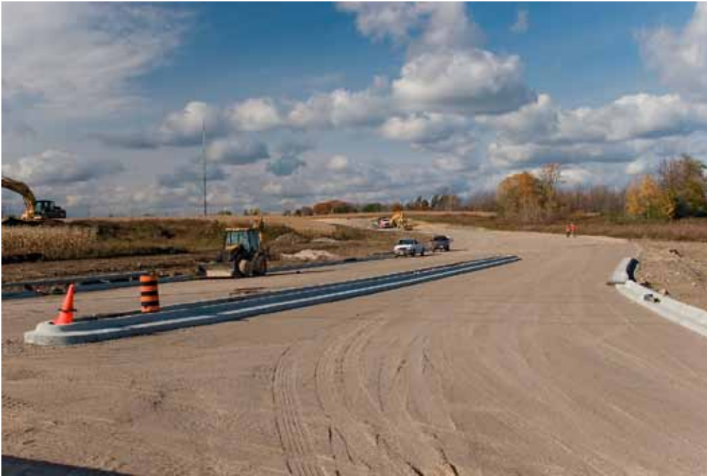
New road construction in developing countries often fails to include space for pedestrians or cyclists – even though walking and cycling are omnipresent travel modes in rural as well as urban areas. (Photo: BigStock)
